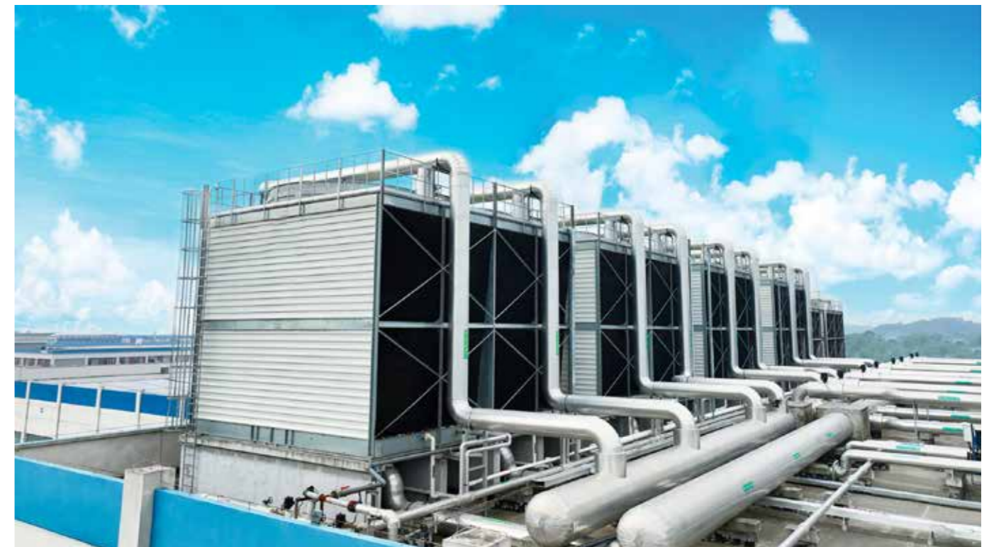
Cooling towers for the solar PV division
