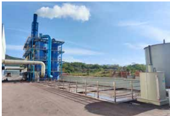
Exhaust treatment facilities of magnetic material furnaces
